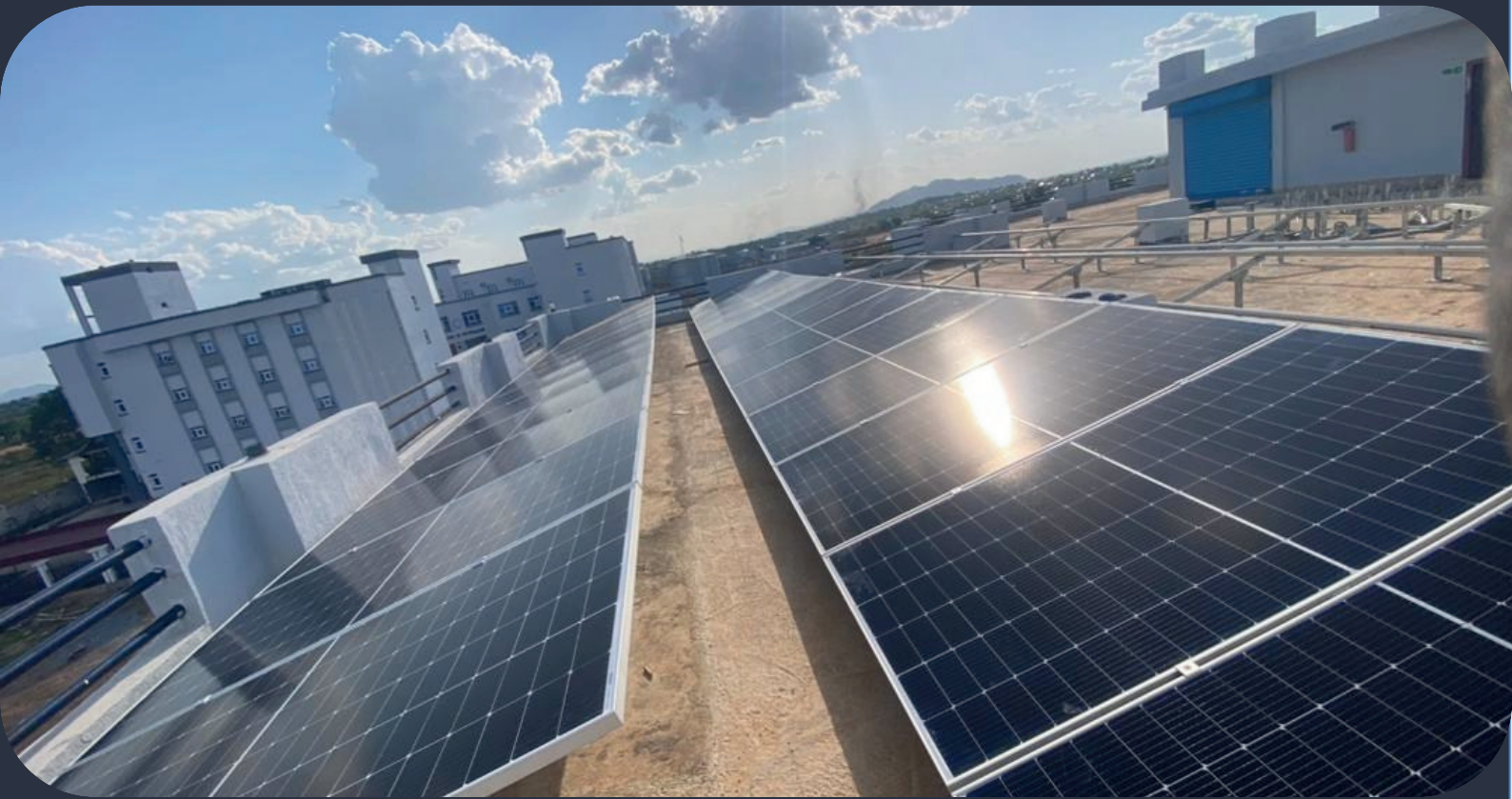
Figure 20: installed solar panels
