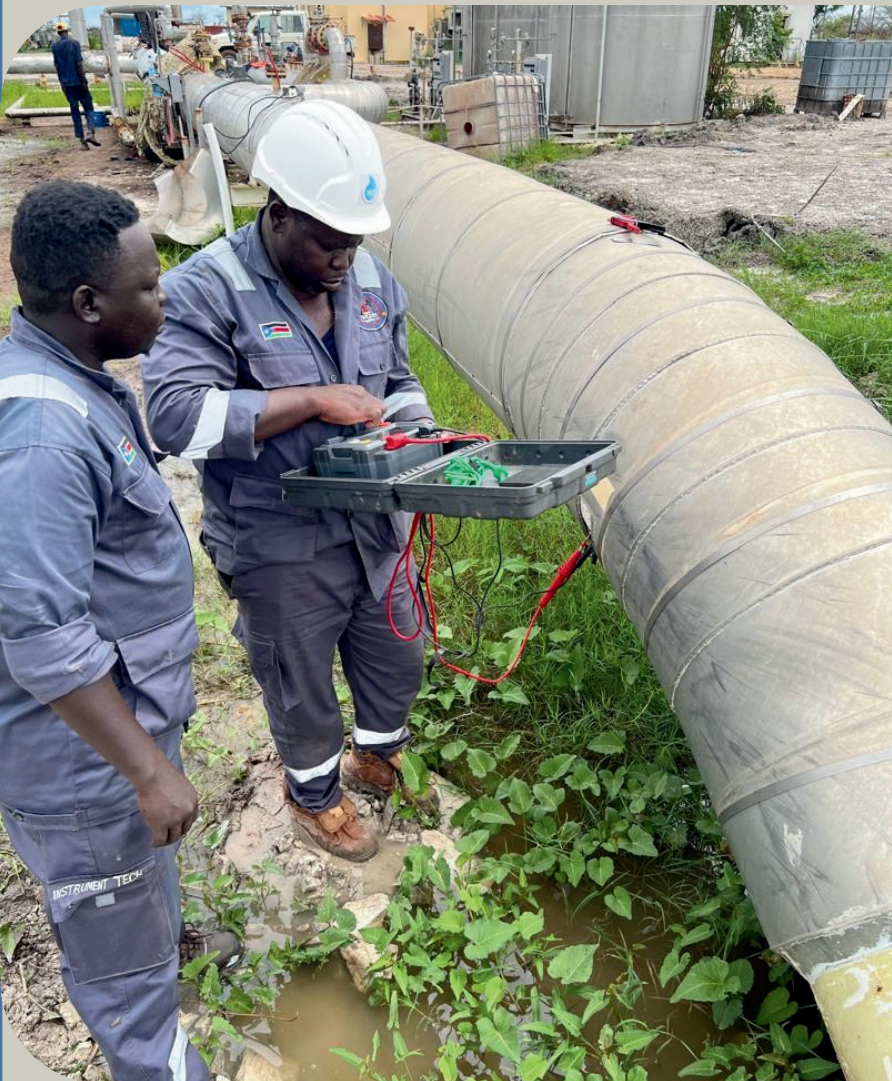
Figure 11: above ground heat tracing
